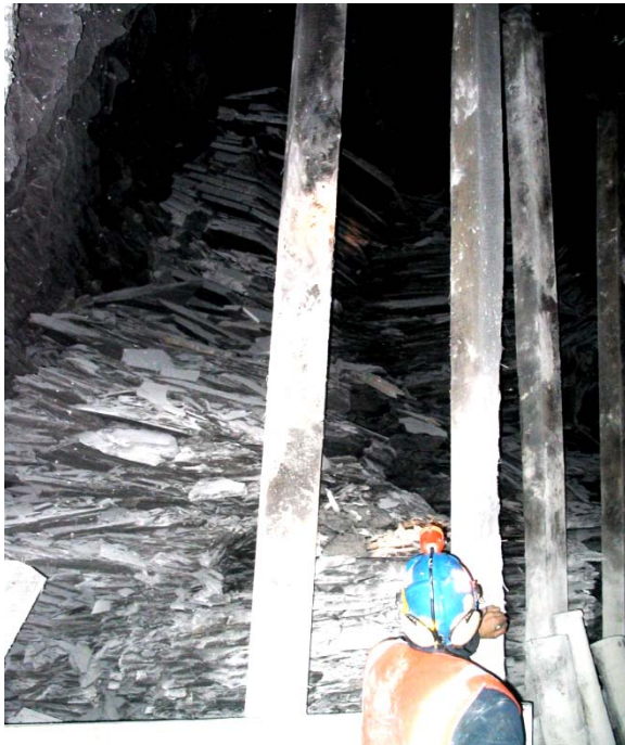
Figure 3: Typical roof fall showing laminated nature of the silty shale roof rocks and steep-sided collapse cavity.
